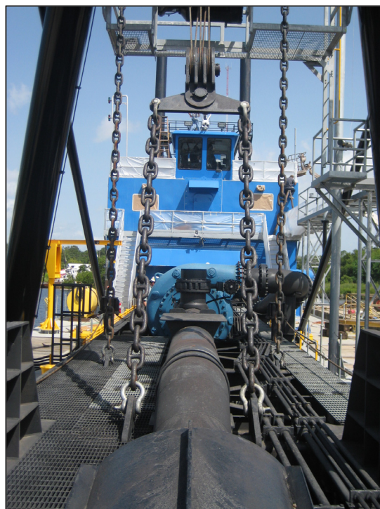
Port of New Orleans' submerged pump dredge being assembled in Slidell, LA.
